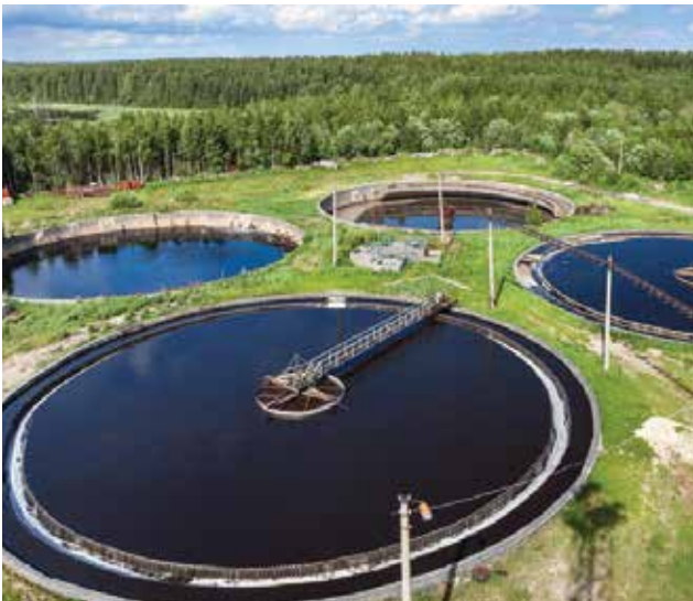
CIVIL AND INDUSTRIAL WASTEWATER TREATMENT
